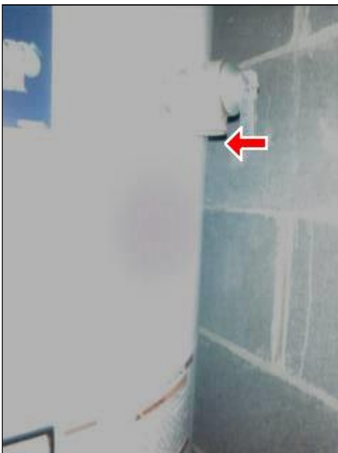
10.6 1 units missing drip tubes
