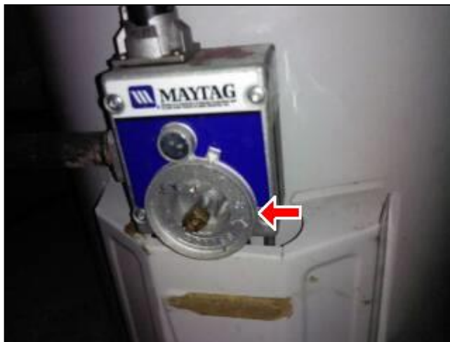
10.6 2 unit #1 missing temp control
