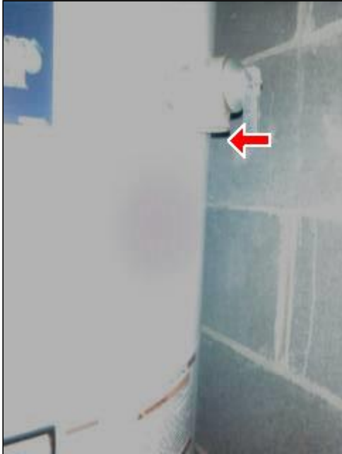
10.6 Picture 1 units missing drip tubes
