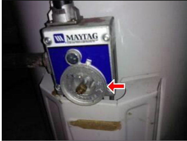
10.6 Picture 2 unit #1 missing temp control
